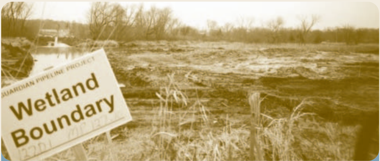
Construction from the Guardian Pipeline Project in the wetlands at the Bank River Crossing in Jefferson County.
